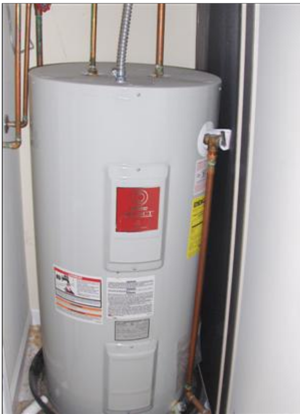
5.2 Picture 1 Water heater.
