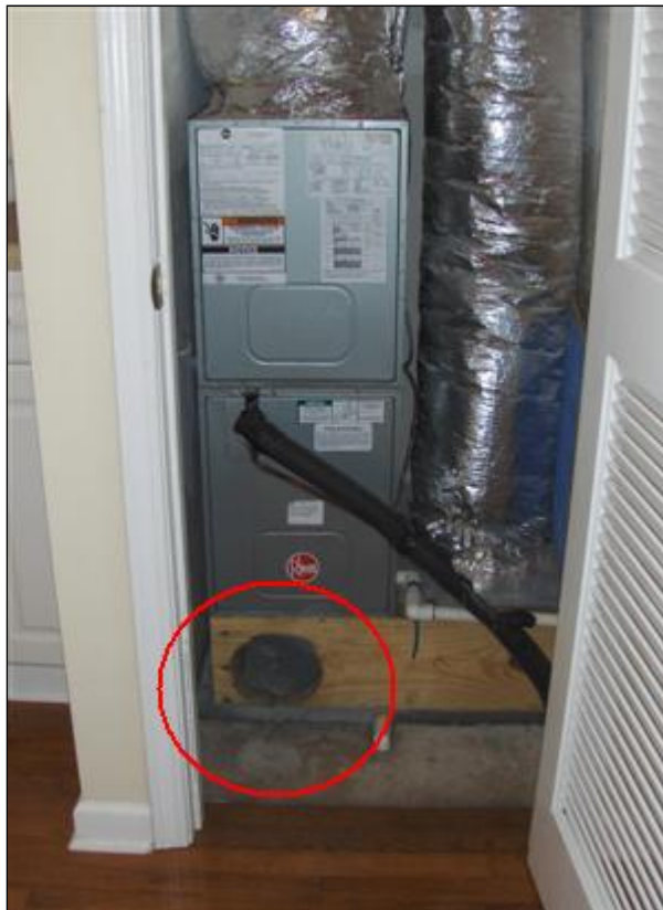
7.3 Picture 1 Mechanical closet.
